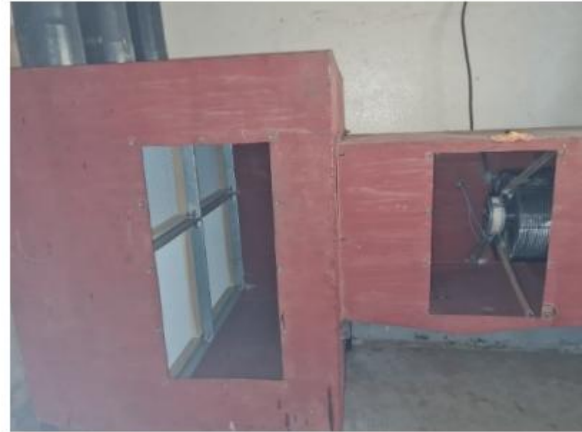
Figure 4: Air system box, with open maintenance doors; H13 filters and radial ventilator visible
