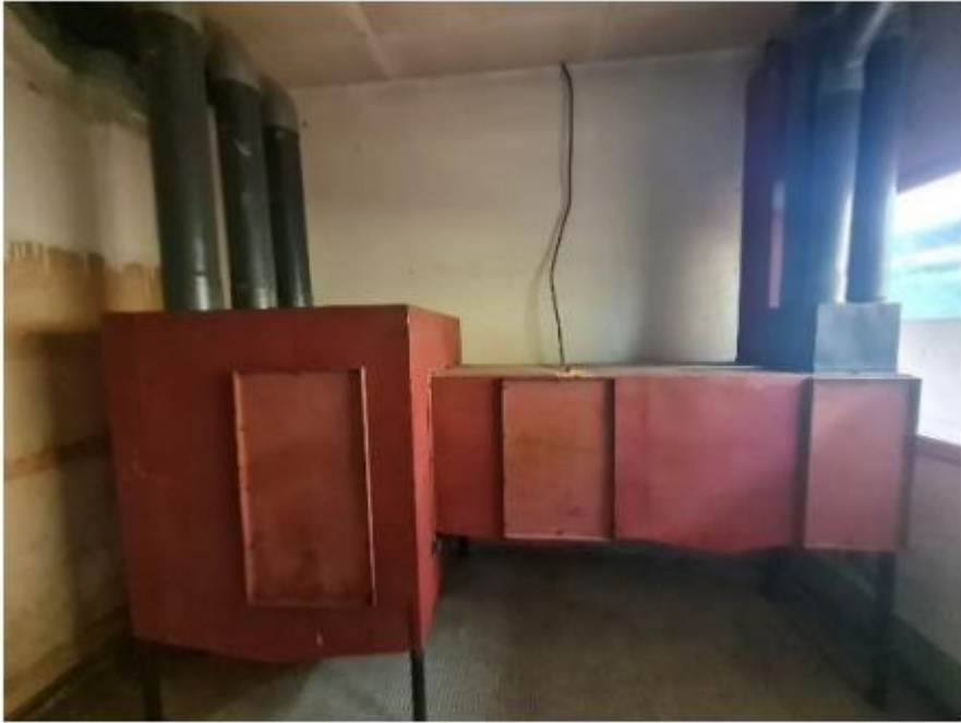
Figure 3: Air system box, with closed maintenance doors
