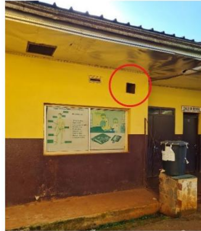
Figure 2: Outside fresh air collector (red circle)
